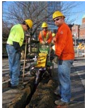
A scene repeated across the country: A construction crew in Memphis, Tennessee, digs a trench along a street for laying a fiber cable.
